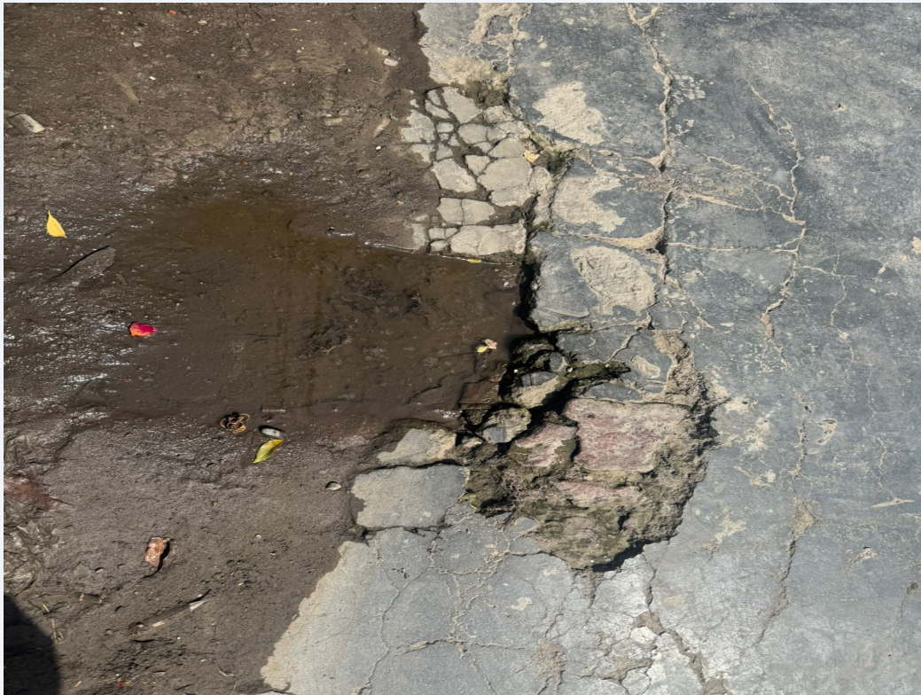
Fig 3 — Close-up of drain boundary: cracked and structurally compromised edge, with water pooling at the paved/unpaved surface transition. Drain unable to contain or direct water flow.
