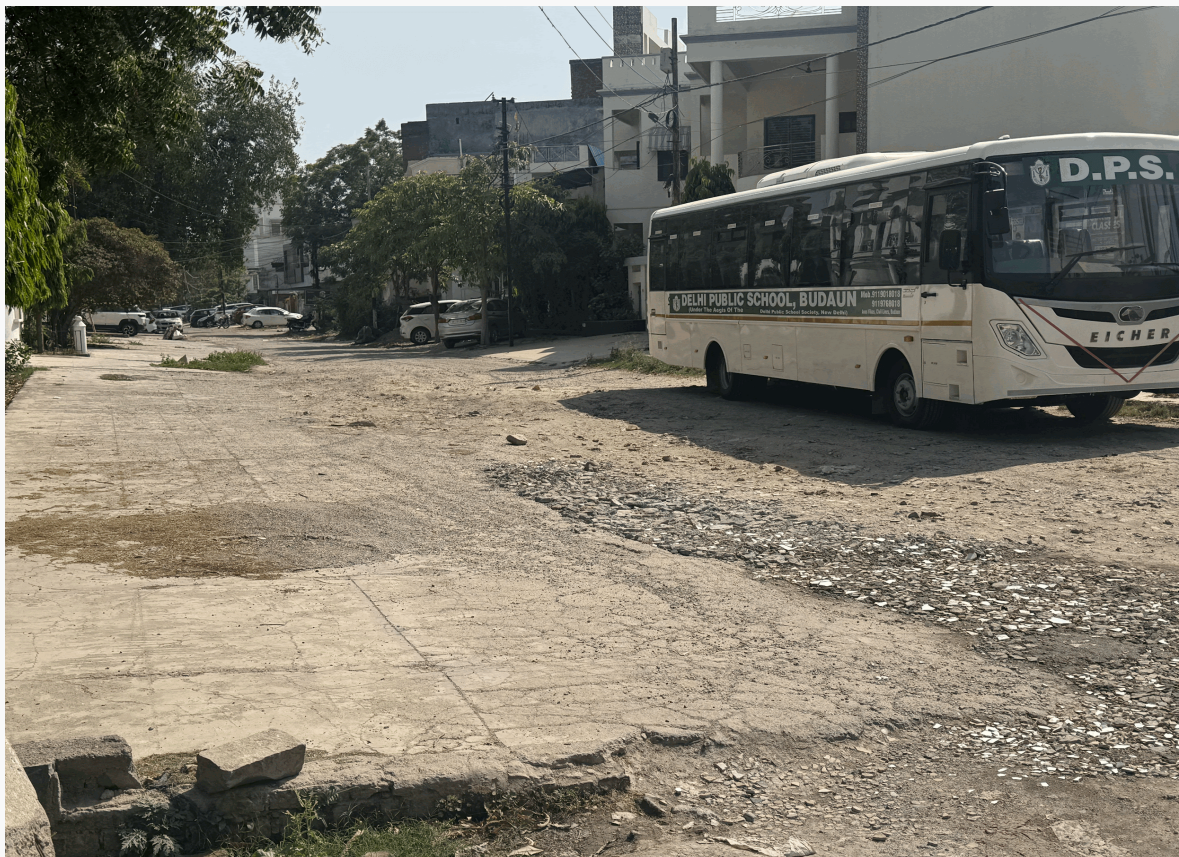
Fig 1 — DPS school bus navigating deteriorated road surface adjacent to Model Town. Gravel displacement and road surface failure visible — consistent with long-term water damage to the road base.
